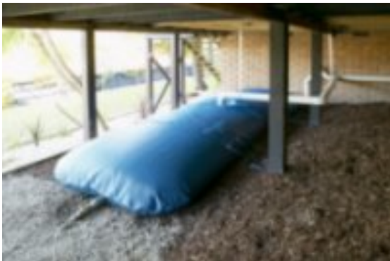
4. Nylex Bladder Tank under a deck
