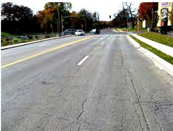
Figure 3.2. Example of asphalt street in fair condition
