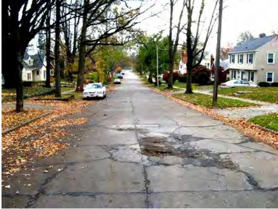
Figure 4.3. Example of concrete street in very poor condition
