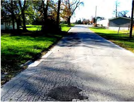
Figure 3.3. Example of asphalt street in very poor condition
